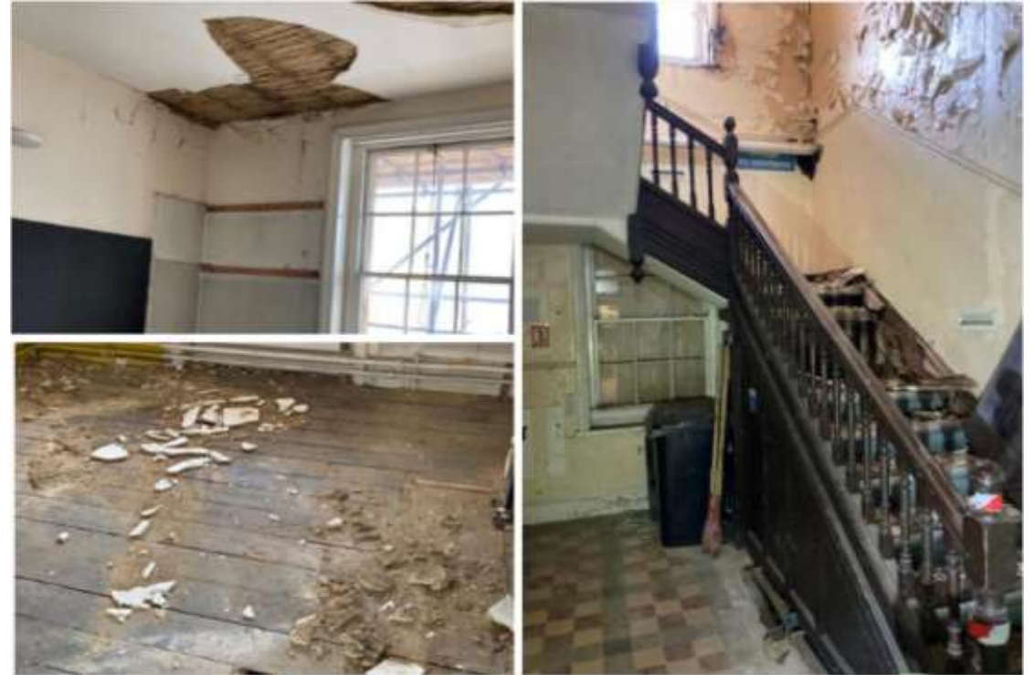
Some of the areas needing repair at Royal Berkshire Hospital (Image: GBS Health)
